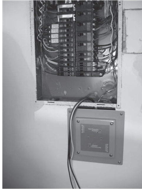
Fig. 5 Sample picture of ground connection to AC panel
