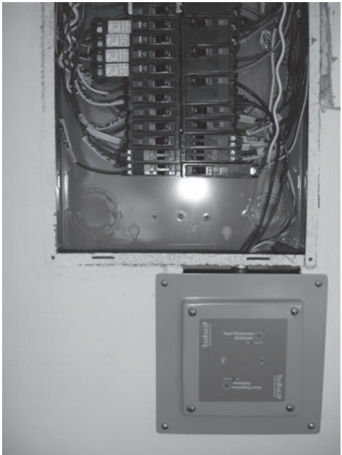
Fig. 6 Sample picture of unit installed and Operating properly
